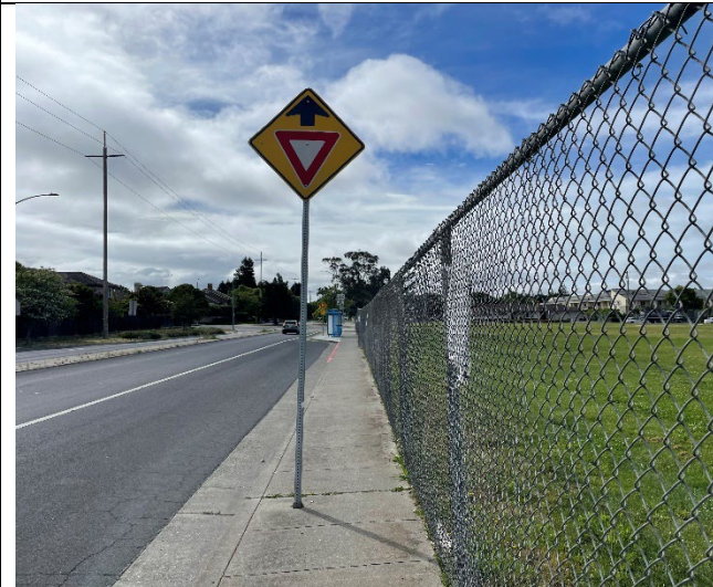
Sign somewhat obstructing sidewalk along Ely Blvd; fencing close to sidewalk
