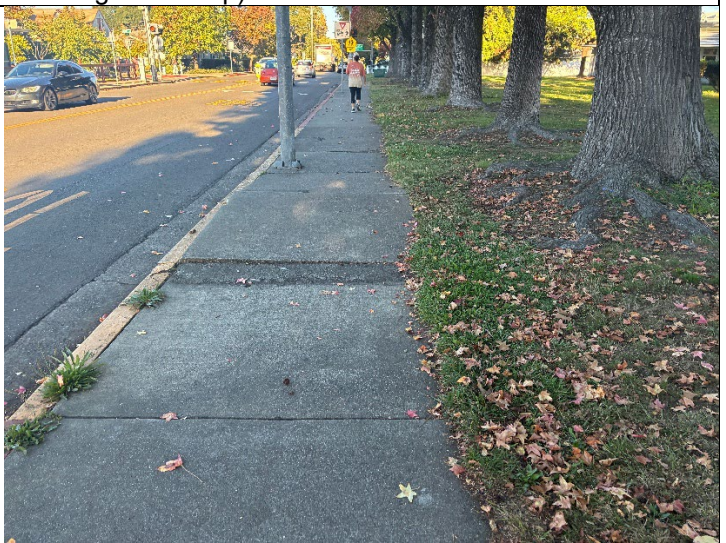
Repair/smooth out lift in sidewalk on Bryden Lane in front of school (cracked due to tree roots)
