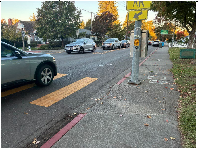
Crosswalk at Bryden Lane & Austin Way (consider widening curb ramp)
